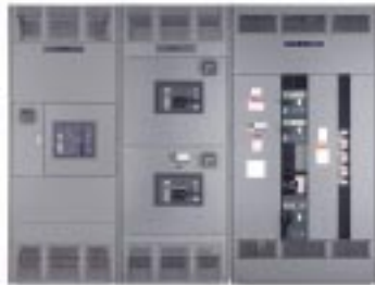
Figure 27: Low voltage switchboard (floor-mounted).
